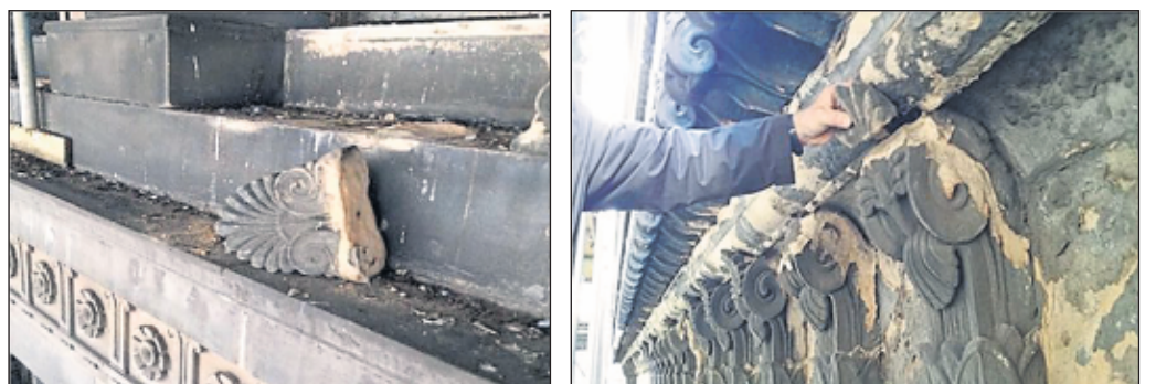
The owners of the Egyptian Halls are concerned about the crumbling masonry on the listed building
